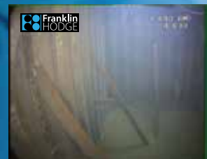
Wall support struts
