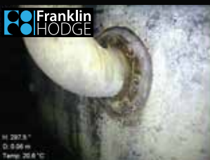
Overflow pipe & connection
