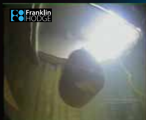
Inlet valve ball float
